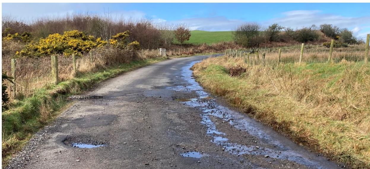
Above: The poor condition of the narrow core path that leads to the site of the proposed solar farm.
